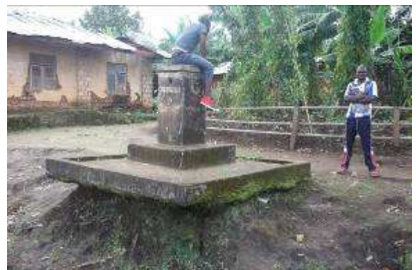
Photo 8.2: Blocked Stand Tap
