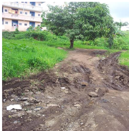
Photo 6 : Way existing access failing
