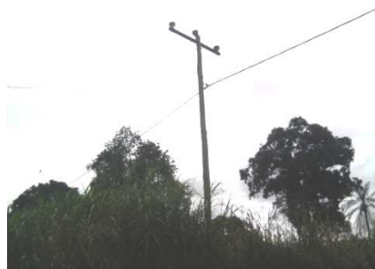
Photo 24: poteau AES/ SONEC
